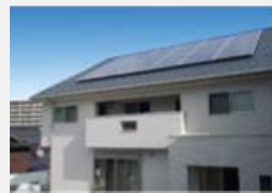
Residential solar power generation system
