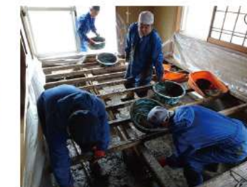
In Toho Village, Fukuoka Prefecture, we provided restoration support such as underfloor mud removal and epidemic prevention disinfection of flooded houses (2017).
